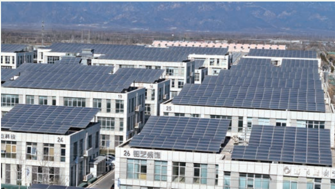
The first photovoltaic power station of Longyuan Power in Beijing was successfully connected to the grid for power generation, which is also the first photovoltaic project both for the CHN Energy put into operation in Beijing
