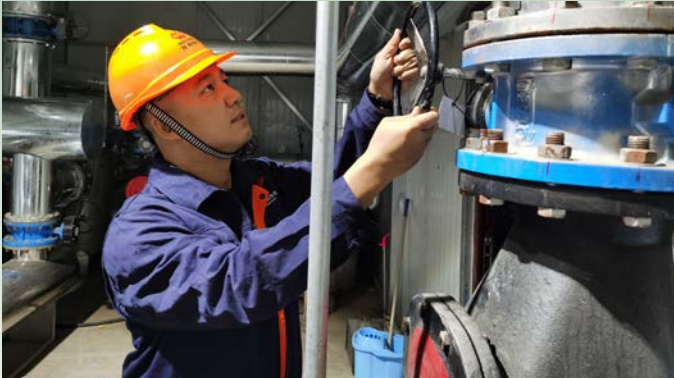
The first heating project with air heat source of Longyuan Power and Xiaonanying heating project being officially started to work
